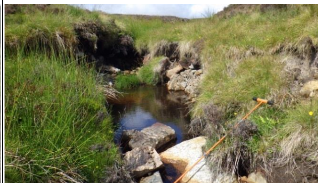
View upstream (east) at NH 3634 6808 showing incised channel with unstable banks and rocky debris.
