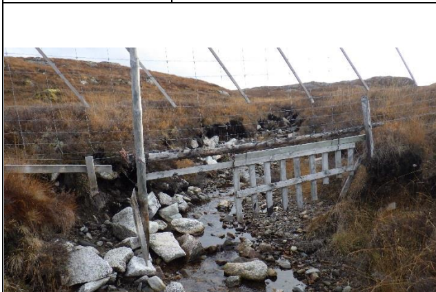
View upstream (south) from NH 3676 6724 showing incised channel with boulder debris and bank instability.
